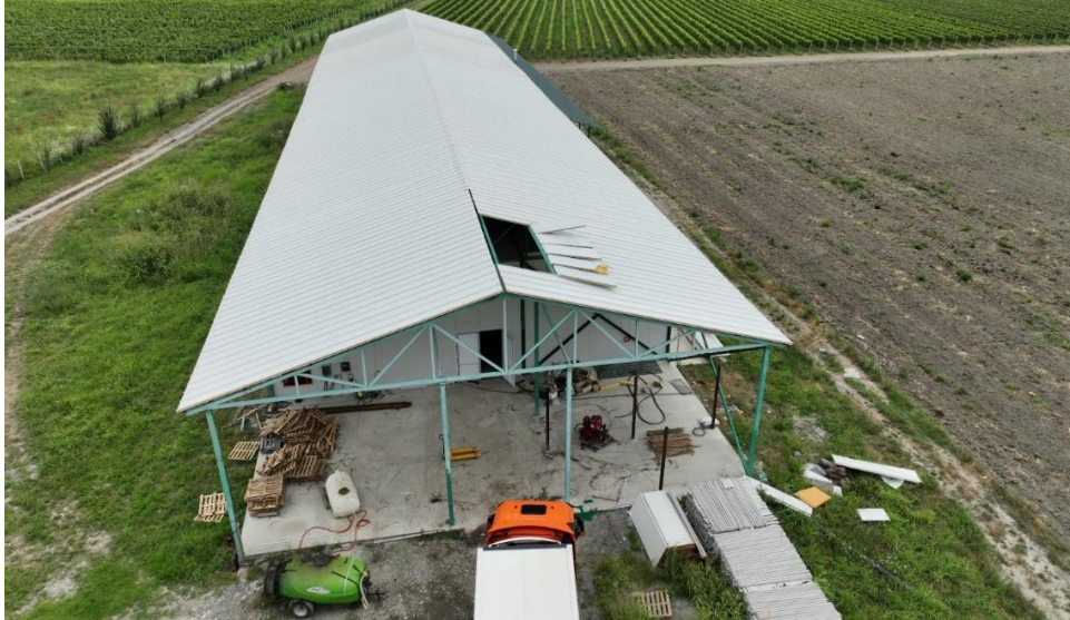
Fig. 8. Agricultural cold storage farm. A part of the building's roof collapsed. Photo from drone. (Point 1, Table 1).
