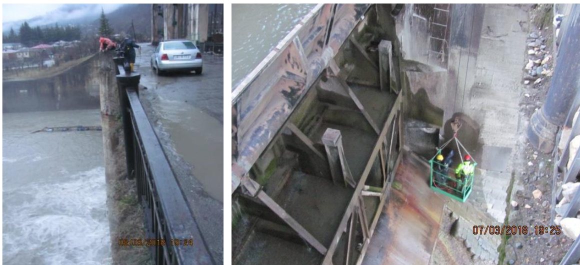
Fig. 8. a) Georadar research process along the second pier (using 1000 MHz antenna), b) low-threshold dam condition investigation process using 1000 MHz antenna.
