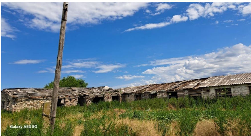
Fig. 7. Farm with badly damaged roof next to the cathedral. (Point 9, Table 1).
